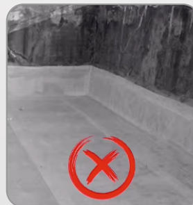
Poor roof waterproofing & thermal insulation performance
