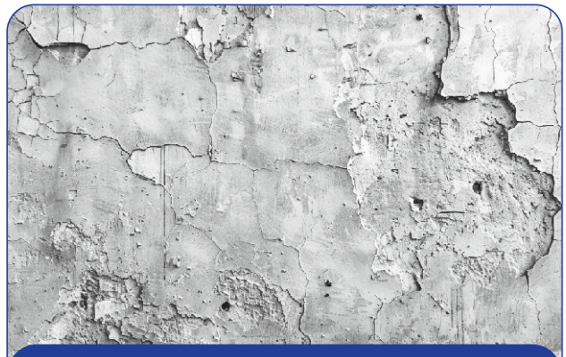
Wall Seepage Crack
