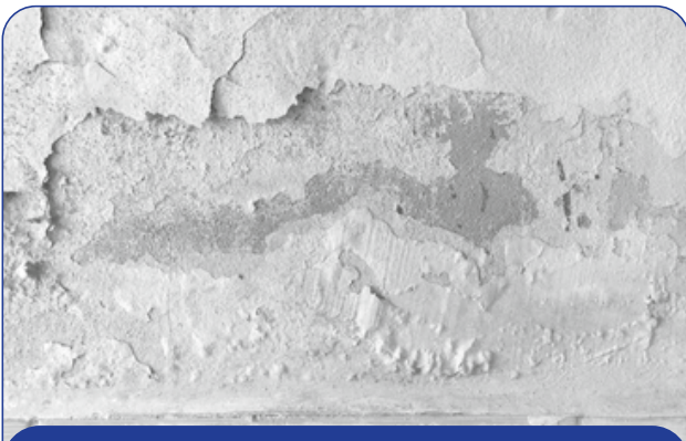
Water Leakage Moldy & Peeling
